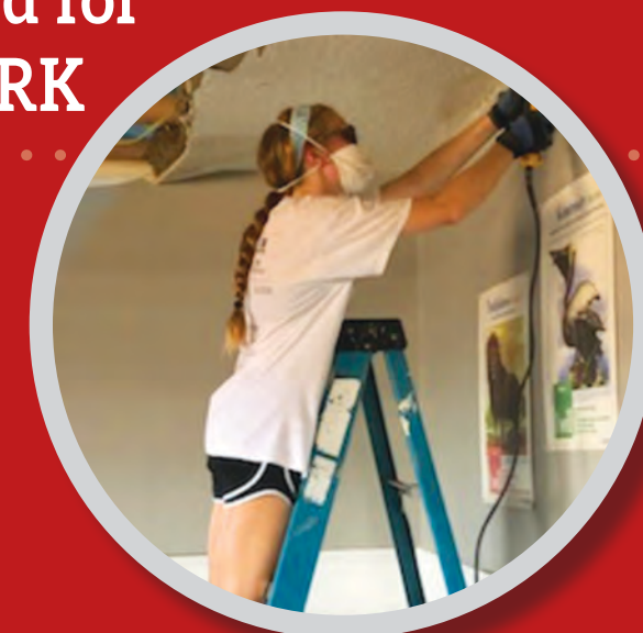
Julia cuts through damaged dry wall from Hurricane Michael in Marianna Florida where she helped rebuild houses.
